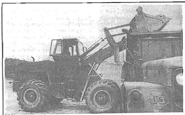
PVT David White of Ashland kept his endloader busy scooping dirt from a Ft. Pickett site and offloading it into a succession of dump trucks while performing construction duties with the 201st Engineers at the Virginia army post.
