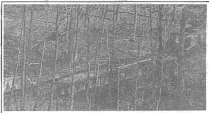
Hidden in the trees, engineers from Co. C, 206th EN BN, set up an armored vehicle launched bridge (AVLB) across a steep gully to accommodate APC's traversing the "battle" area. (Photo by CW2 James D. Pope Jr., 133rd PAD)
