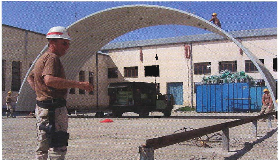
Command Sgt. Maj. Greg Armstrong oversees the construction on the Afghan National Army's Warehouse Depot Office Building in Kabul, Afghanistan, April 1. (Photo by Staff Sgt. Kelly McCargo released).
