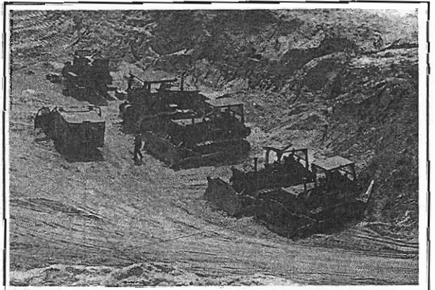
Members of the 201st Engineer Battalion of the Kentucky Army National Guard worked around the clock for nearly ten days during their recent annual training period here to repair and improve a tactical airstrip on this 72,000-acre post in North Florida. Bulldozers and other vehicles are shown here in the "borrow pit" where clay was excavated for the runway surface. (Photo by CDT Sallie R. Boward)
