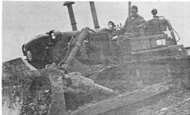
GUARD SERVICE - SP5 Donald L. Morrison, of the 207th Engineer Company, pushes dirt over a portion of a "sink hole" in Brandenburg as a disposal area for debris collected after the April 1974 tornadoes. About 3,000 square yards of dirt were used to help the community eliminate a health hazard. (Photo by SP4 Frank Lauyans)
