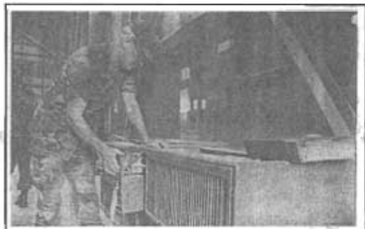
SSG William Allen searches for wiring problems in a 36,000 BTU heat pump at a Fort Knox maintenance facility.
