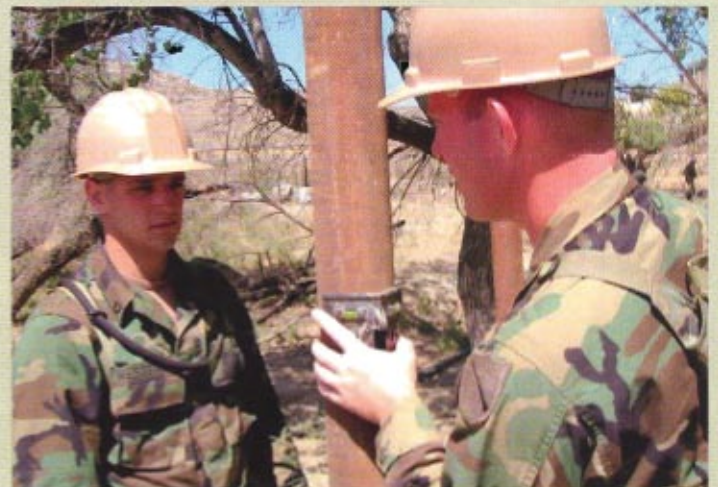
Pfc. Daniel Westfal and Sgt. Jason Earley level posts prior to installing the barrier fence.
