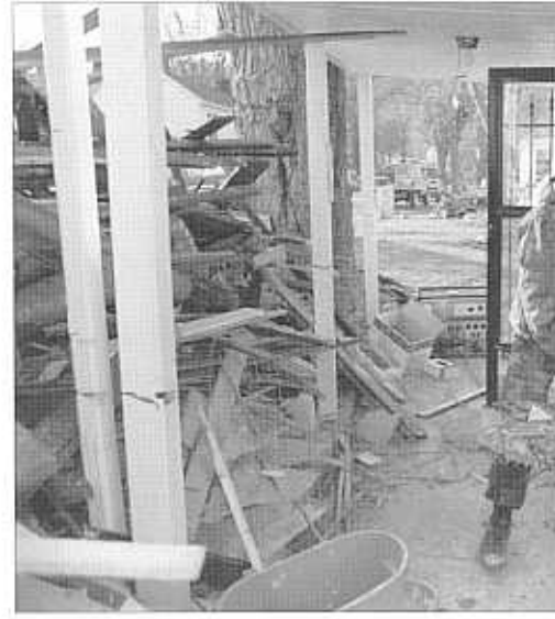
ABOVE: Staff Sgt. Darryl Brown of the 123rd Medical Squadron uses a shovel to clear debris from a home in Owen Sound.
