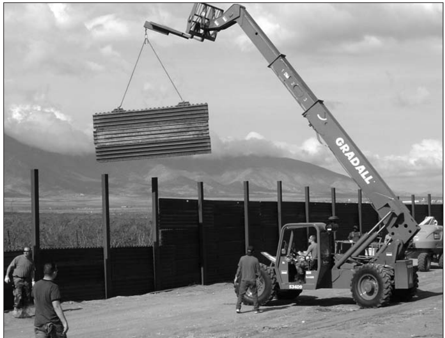
Above: Airmen position the steel matting to extend fencing between the United States and Mexico.
