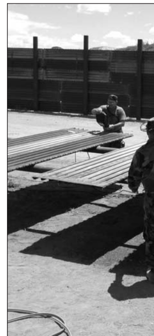
Above: KyANG civil engineering members work on a steel fence in Bisbee, Arizona.
