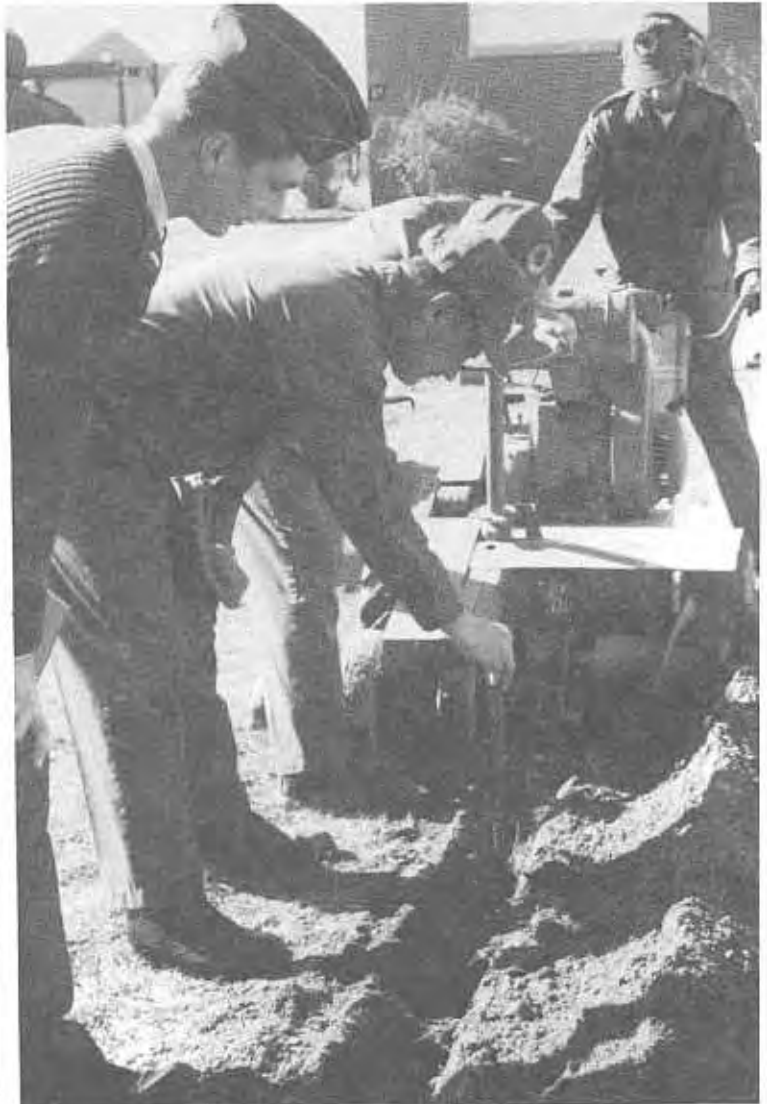
From left, 2nd Lt Phillip Howard, TSgt. Joseph Cslank, SrA Michael Coryell, and SSgt. Jimmie Spann, 123d Civil Engineering Squadron, dig a ditch to install a communications cable for a computer link up.
