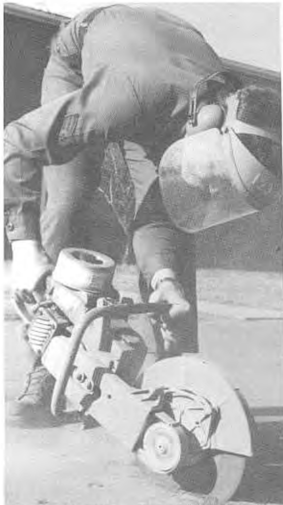
Sgt. Gordon Stacy, 123d Civil Engineering Squadron, cuts into a road, preparing for installation of a communications line.
