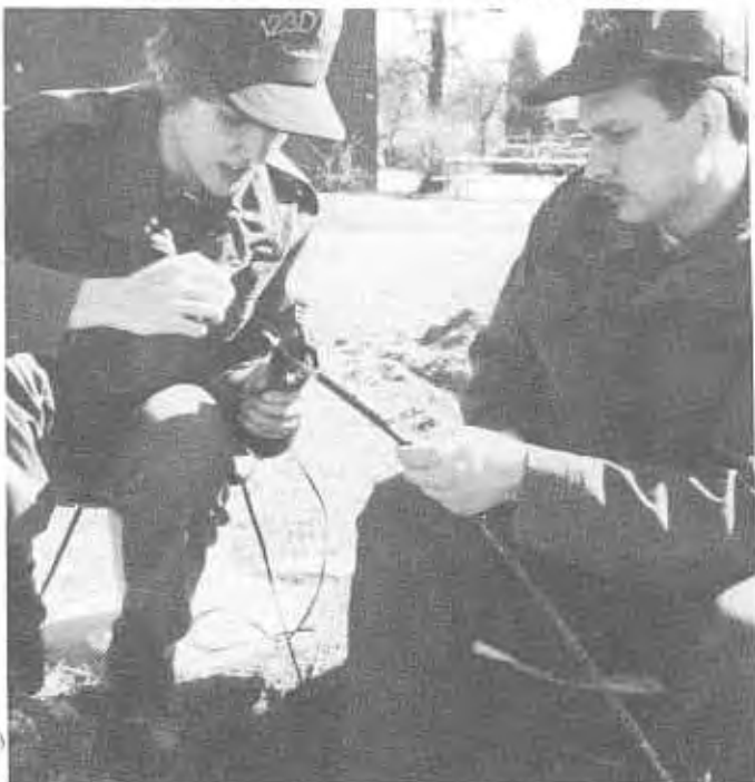
SrA Bettina Schwallie and SSgt. Richard Stradley, 123d Communications Flight, repair a cable for the base CCTV line.
