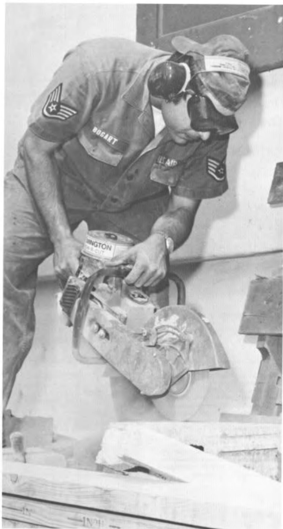
CE IN PUERTO RICO: SSgt Bruce Bogart cuts a concrete block during a 1974 project which took the 123d Civil Engineer Flight to Ramey AFB, Puerto Rico. The Engineers were becoming widely recognized and much in demand for their skills, but pulling field training in Puerto Rico wasn't so bad on their own morale as a unit, either.
